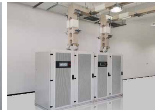
Winter Olympics 200kW/100kWh project
