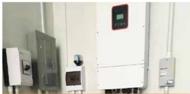
Jamaica 7kW/20kWh residential ESS project
