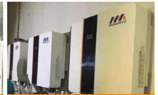
Greece 5kW/10kWh residential ESS project
