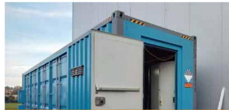
250kW/630kWh C&I ESS project in Austria
