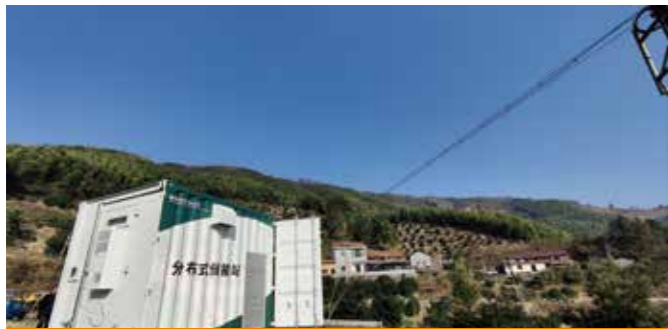
250kW/200kWh microgrid project of Zhejiang
