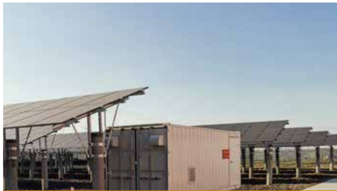
Nanjing 150kW/200kWh microgrid Project
