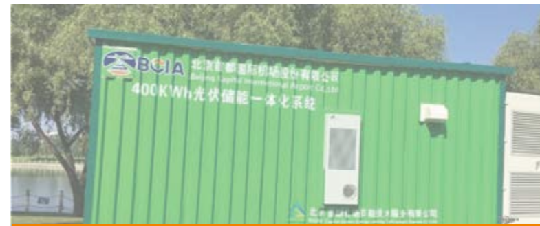
Beijing Capital Airport 100kW/430kWh hybrid project
