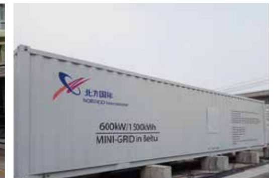
Ethiopia 600kW/1500kWh ESS project
