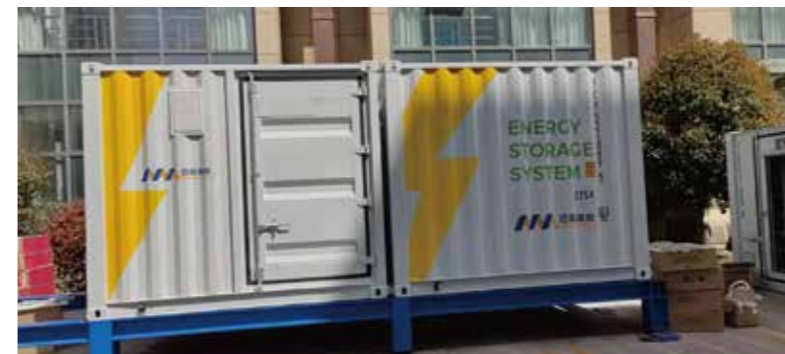
Pakistan 150kW/306kWh microgrid project
